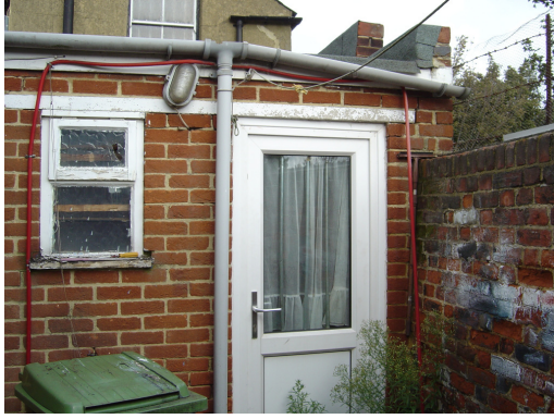
Plate 5 Rear ground floor door to be replaced with part glazed timber door.
